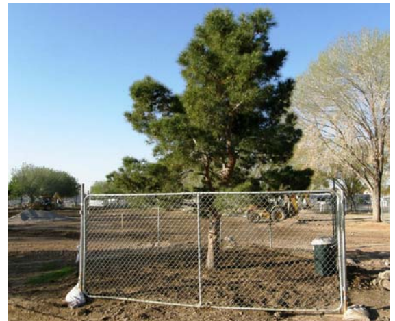
Protecting the root zone of a tree before construction begins is the best way to prevent soil compaction. All photos courtesy: Russ Thompson
