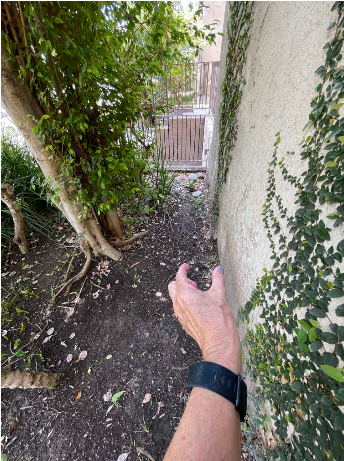
PHOTO - Ficus benjamina - This tree is near a foundation wall. Exploratory trenching should be performed on back of tree, near wall, and roots examined and possibly root pruned, and a root barrier installed to reduce impact from the massive Ficus roots.
